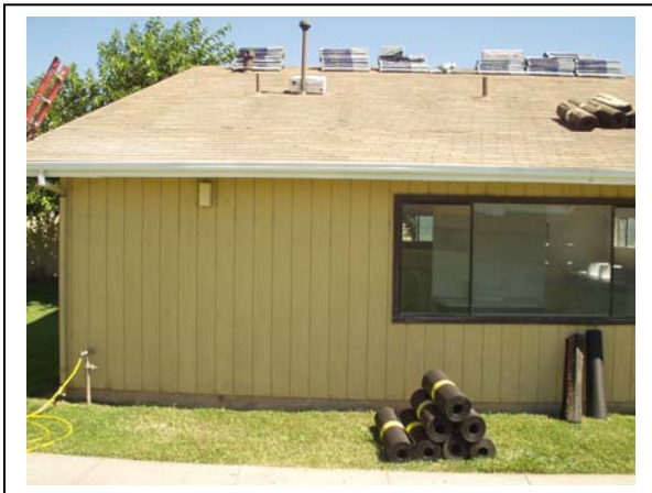
Old roof, windows and exterior paint
